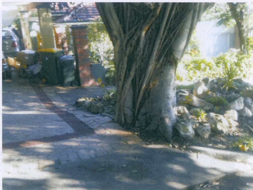
Figure 2 shows trunk in location to driveway.
