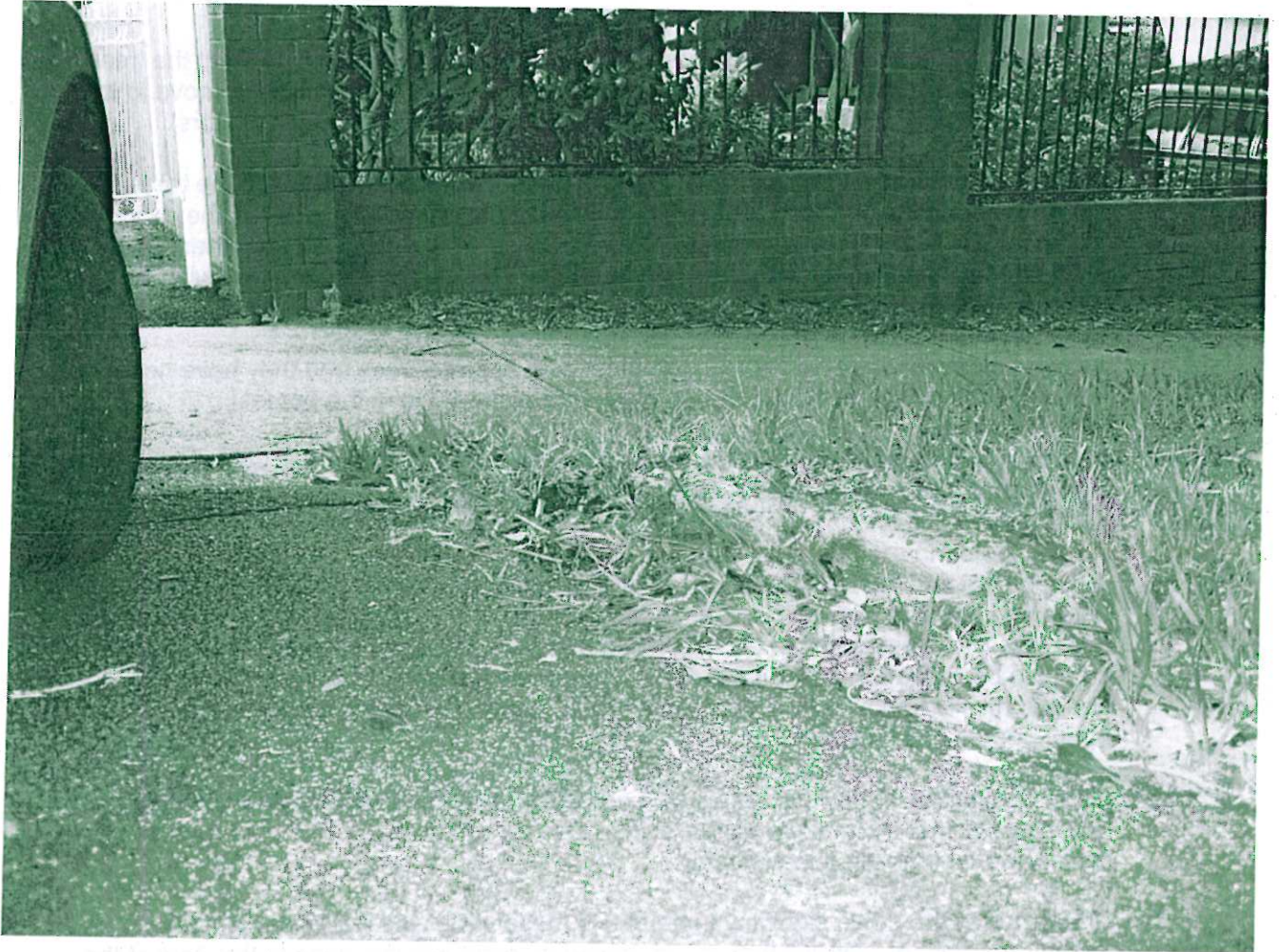
Photo 1. Raised roots, approximately 12 inches above ground and rising!
